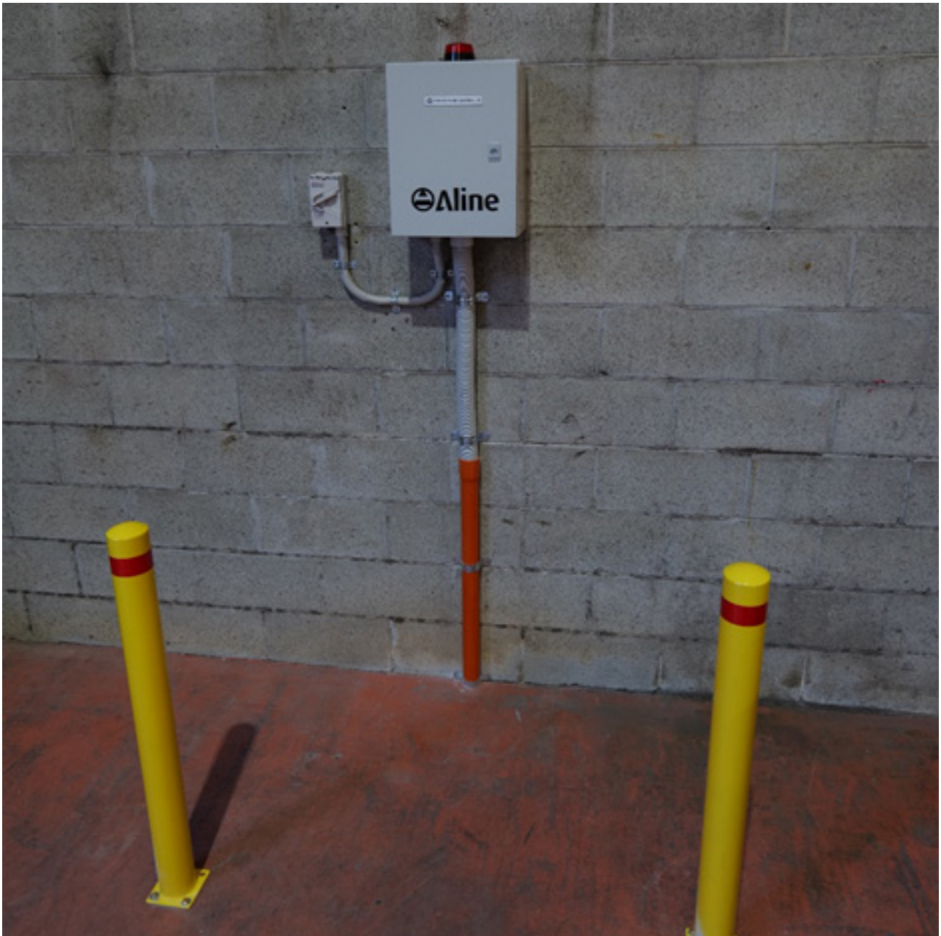
Example photo demonstrating the compliant conduit configuration in a non-UV radiation exposed area.
